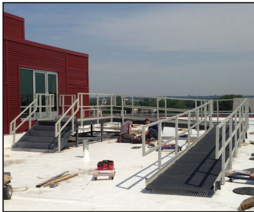
Some sections of the platform were fabricated on the ground before being lifted to the rooftop.
